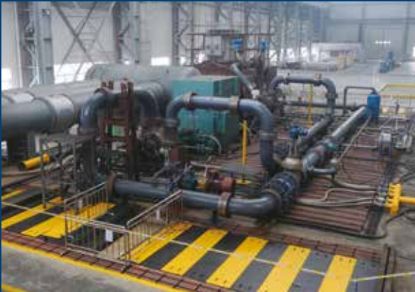
Test Bench for Large Pump 大泵试验台
