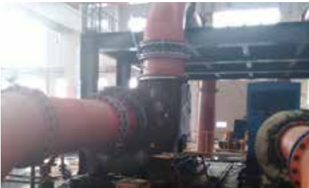
• Test of the desulfurization pump with the diameter of 800 800 口径脱硫泵测试
